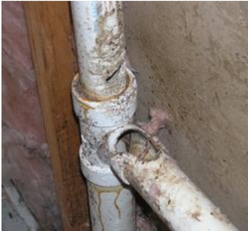
Plastic drain pipes chewed through by rats
